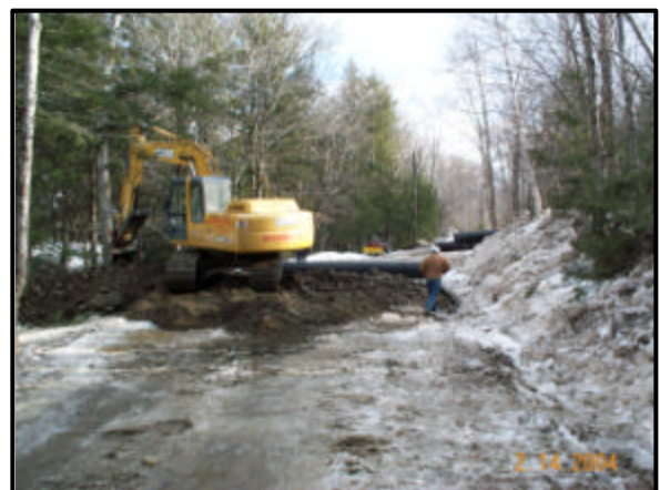
Many cubic yards of ice were removed and piled near the road before culvert installation.
